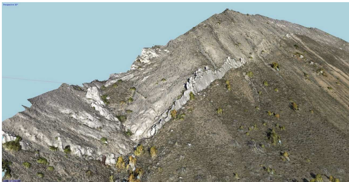
Figure 1: SfM-derived dense cloud acquired from a helikite: a portion of the Roccapreturo bedrock fault plane (Central Italy).
