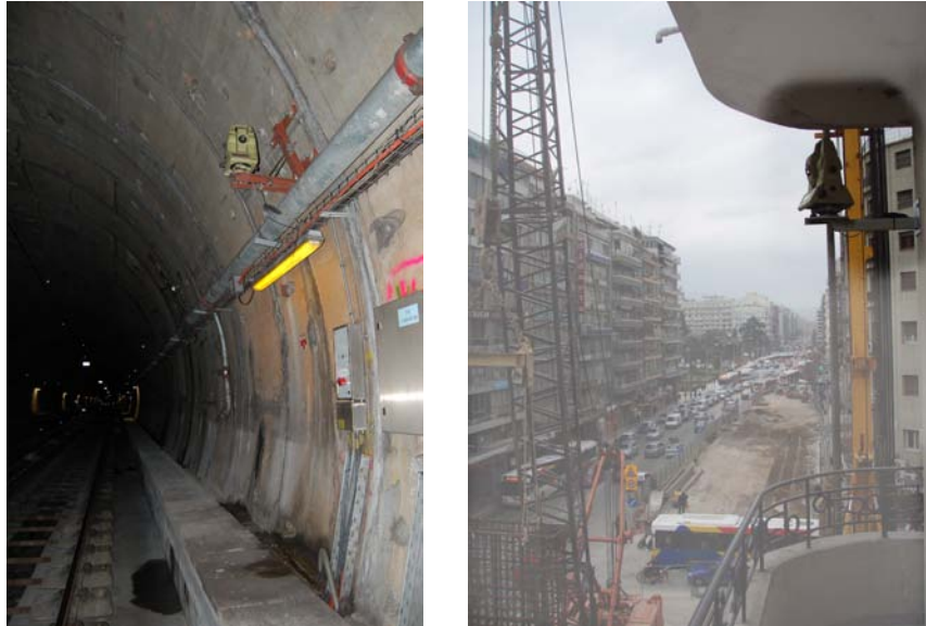
Figure 4: Online totalstations monitoring deformations underground and on the surface.
